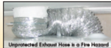
Unprotected Exhaust Hose is a Fire Hazard
